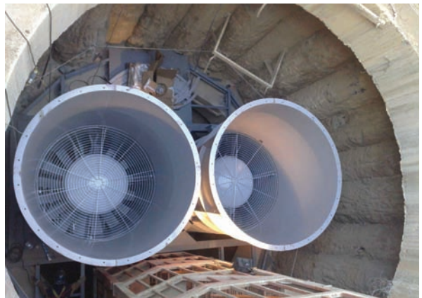
Calle-30 bypass tunnel (Madrid) exhaust vertical fans: diameter 2,800 mm power per unit 630 KW
